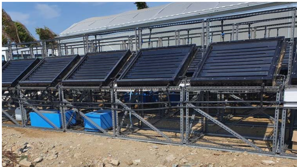
FIGURE 22 Low-cost solar driven desalination system in Tinos (Source: www.hydrousa.org )
